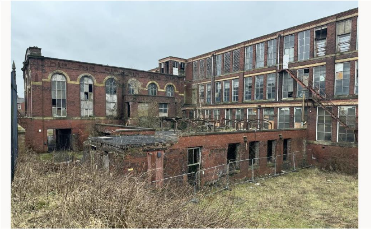
Figure 12 – Photograph of Boiler House adjoining the Engine House and main Mill behind
